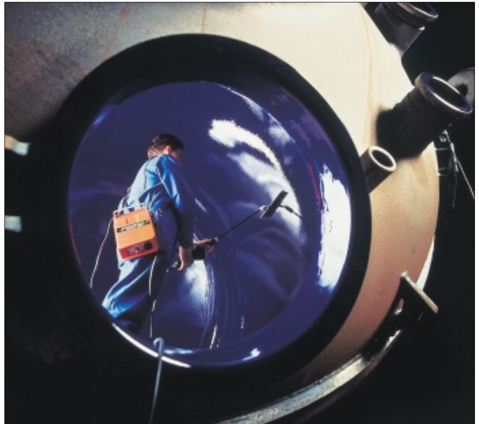
Pore testing the enamel coating of a boiler using the POROSCOPE® HV20.
